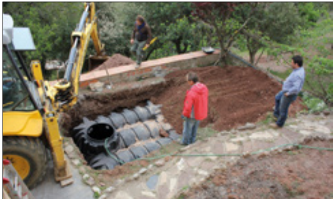
3,500 l (925 US gal.), Building, Vacarisses (Spain)
