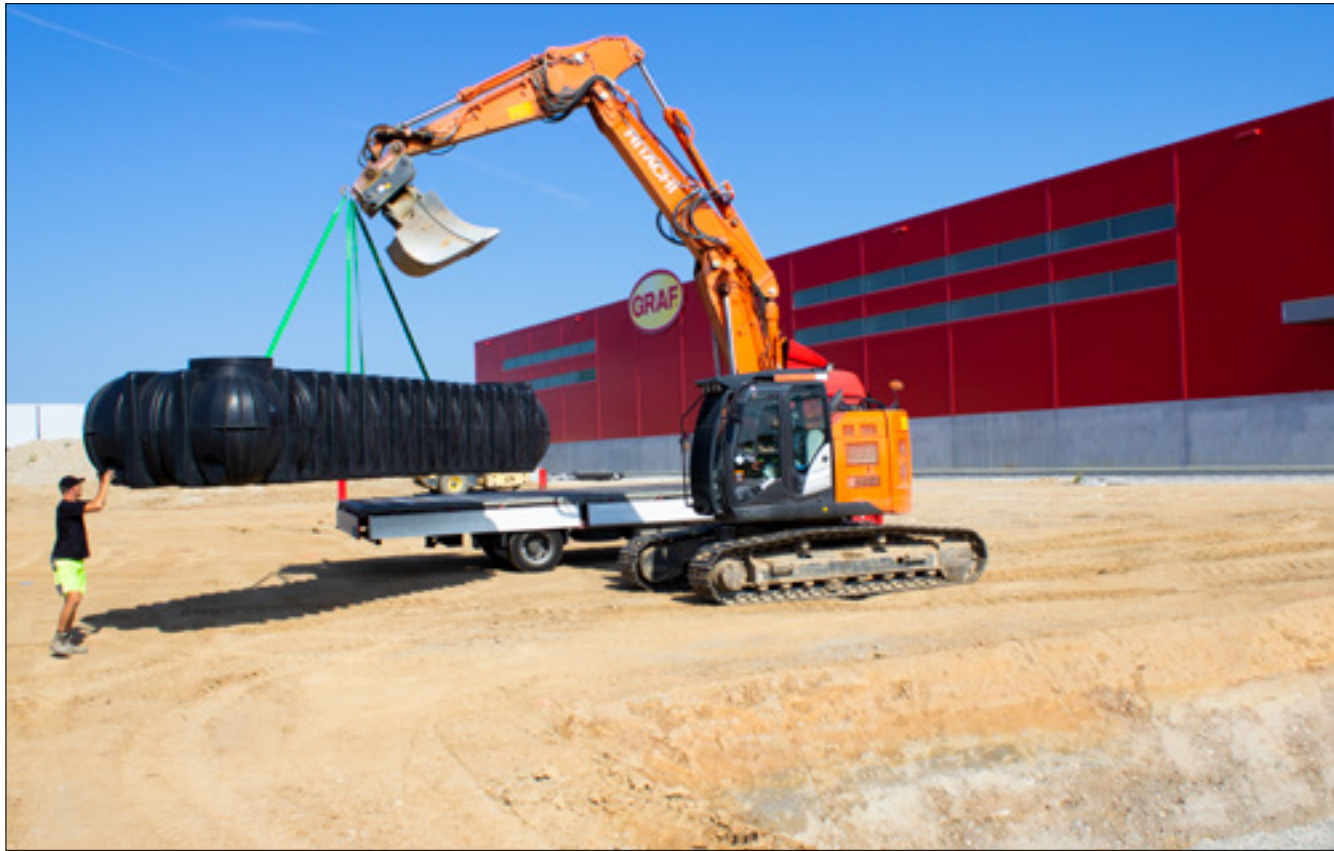
15,000 l ( 3,960 US gal.), Production plant, Herbolzheim (Germany)
