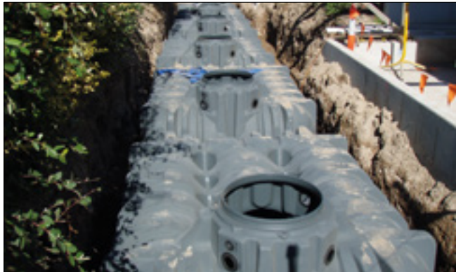
30,000 l (7,926 US gal.), Industrial plant, Geelong (Australia)
